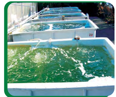
Tanks with vigorous aeration
